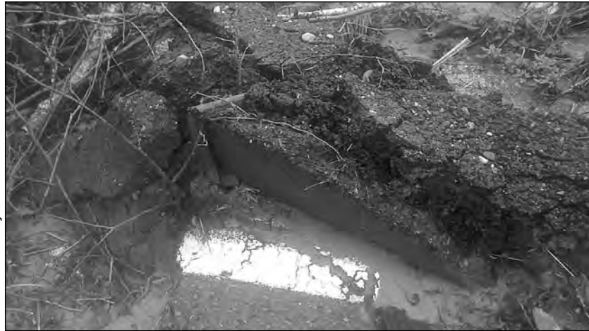
Illahee Road asphalt paving, here showing the white center-line stripe, washed into Gilberton Creek.
