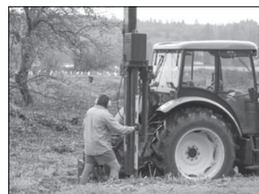
Jade Pope of Jade Agritech, LLC installs a new exclusion fence on the Klingel Wetland.
